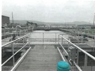
Domestic Aeration Basin
