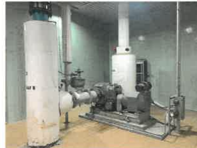
Aging Domestic Aeration Basin blower
