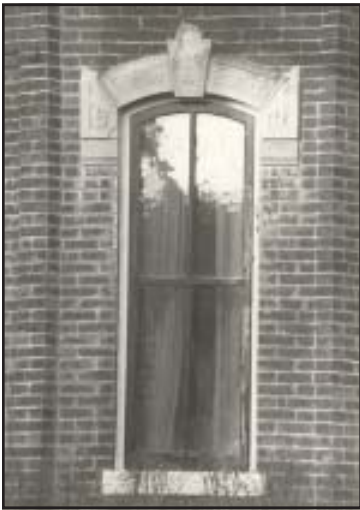
Window detail of the Chesley Mossman house, 619 S. 13th Street. (Photo courtesy of Roger Martin.)
