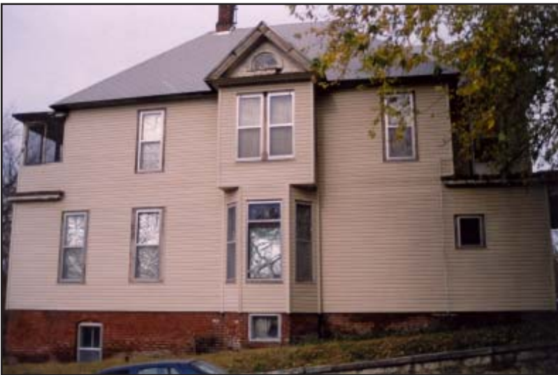
Vinyl siding is installed on this N. 9 th Street Queen Anne house resulting in the obscuring of decorative shingles and wood panels in the bay window area.
