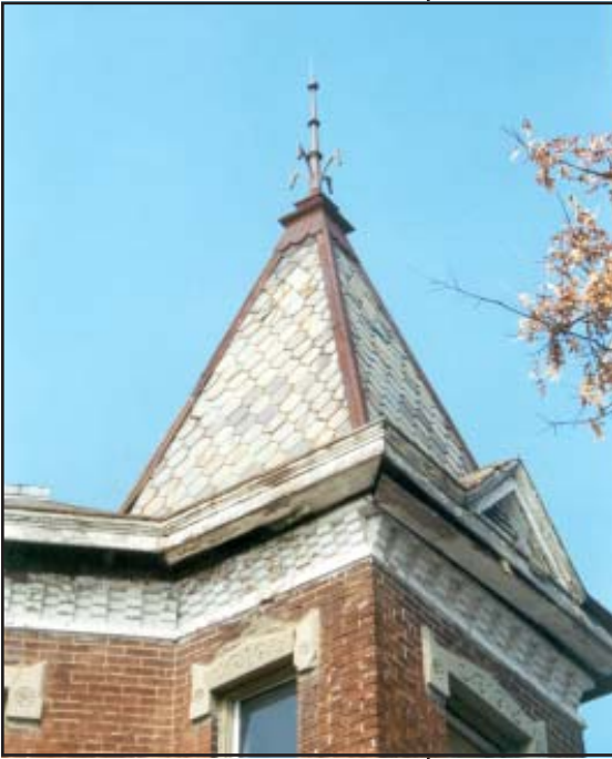
Built-in guttering failure often leads to soffit and eave damage if not corrected. Despite the deterioration, note the intact hexagonal slate tiles, metal ridging, and finial on the tower of the Louis Stigers house, 1023 Church Street, Cathedral Hill Historic District.
