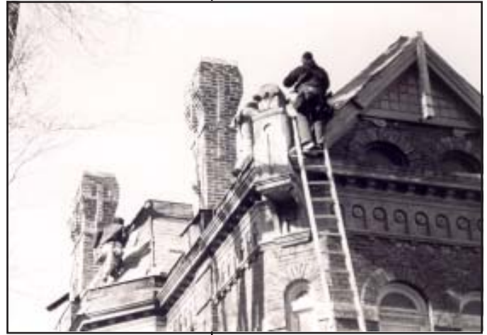
Workers install new slate shingles on the roof of the John Shireman, Jr. house, 120 S. 15 th Street, Museum Hill Historic District.
