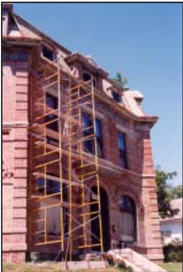
Restoration work is underway at the Joseph Corby mansion, 302 S. 11 th Street, Museum Hill Historic District.
