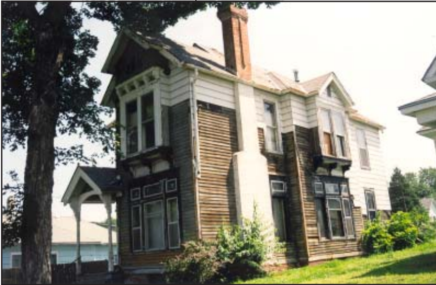
Removal of asbestos shingles on the 1890 Thomas Rogers house, 913 N. 12 th Street, Cathedral Hill Historic District, reveals the original wood siding and decorative detailing. Removal of inappropriate later siding is classified as a 'minor works' item.
