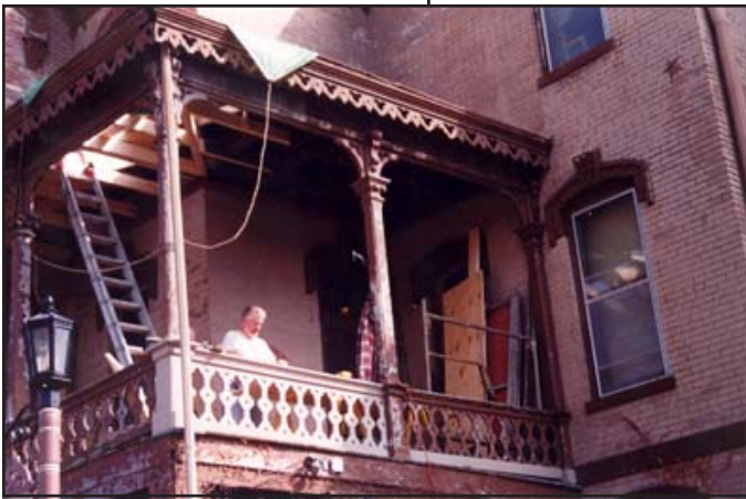
Contractor Ron Petersen repairs the Italianate side porch of the Browne-Craig mansion, 402 S. 12th Street, Museum Hill Historic District.
