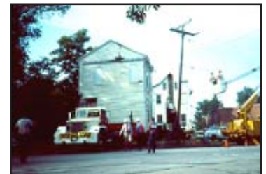
Relocation of a historic building should be a last resort to demolition.
