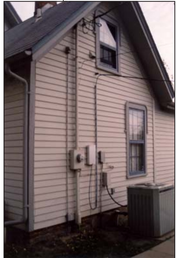
Paint meter boxes and other utility connections in colors that blend with the color scheme of the building.
