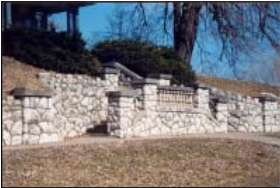
Coursed ashlar retaining walls (top) consist of regularly shaped stone blocks of the same size that provide continuous horizontal joints. Random rubble retaining walls (bottom) consist of irregular, randomly dimensioned natural stones laid without continuous mortar joints.
