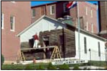
Painters apply a primer coat to the Jesse James House during its restoration in Patee Town. (Courtesy: St. Joseph Department of Planning & Community Services)
