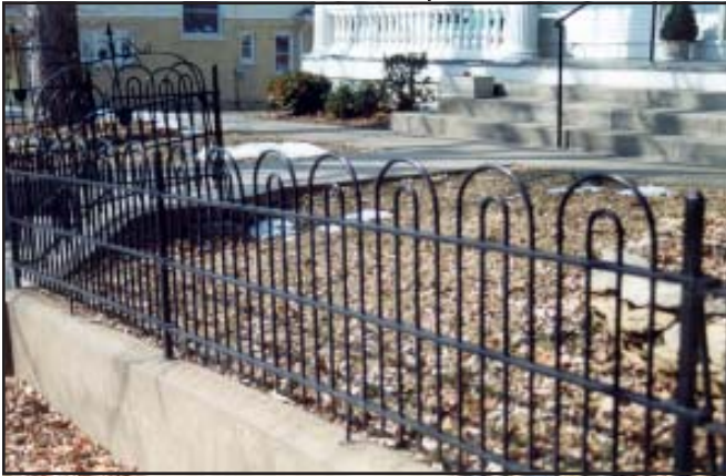
Maintaining a sound paint layer on metal surfaces is essential for preventing rust and corrosion caused by exposure to the weather.
