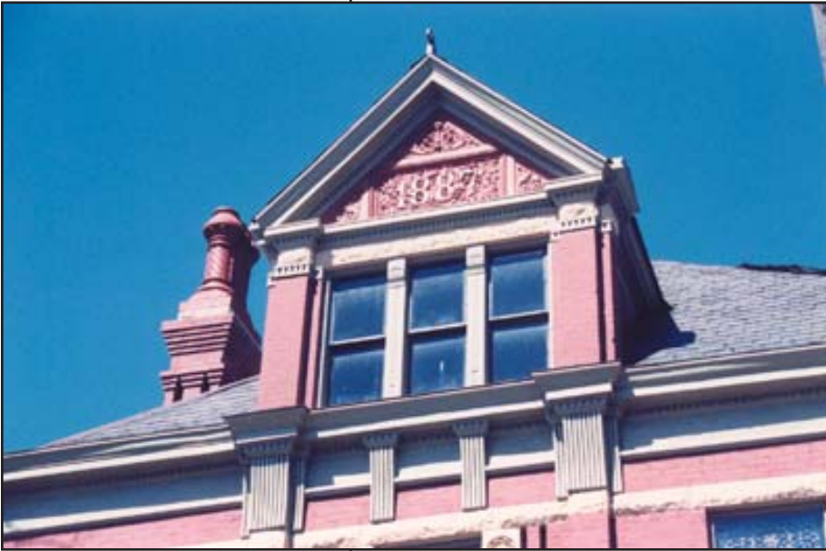
Terra cotta stone inscribed with the date "1887" embellishes the front dormer of the August Nunning house, 1401 Jules Street, Museum Hill Historic District.
