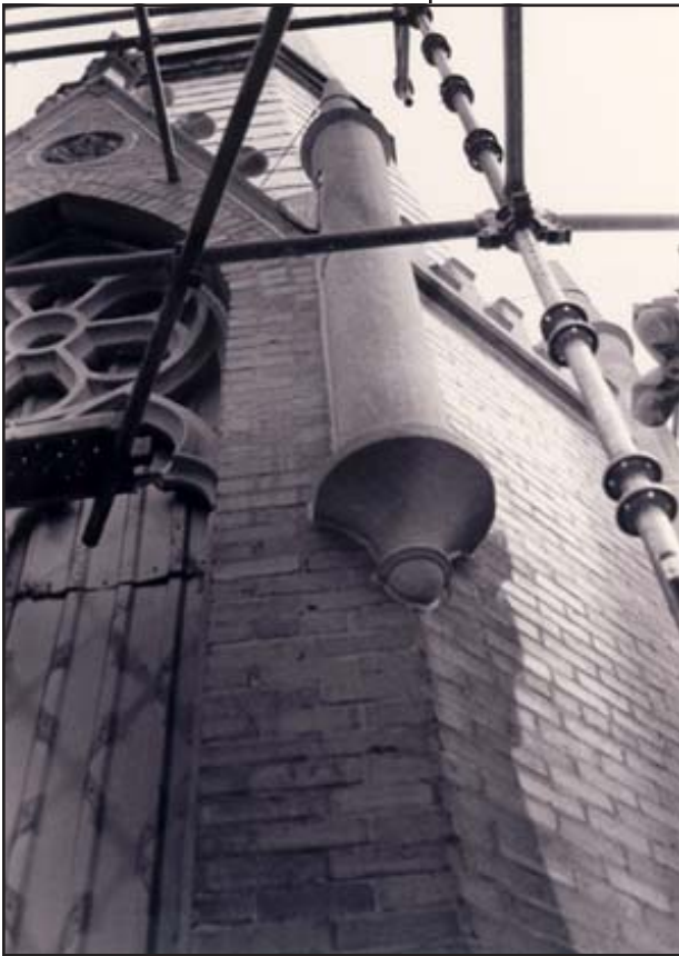
Masonry restoration occurs at Twin Spires Museum, 501 S. 10th Street, Museum Hill Historic District.
