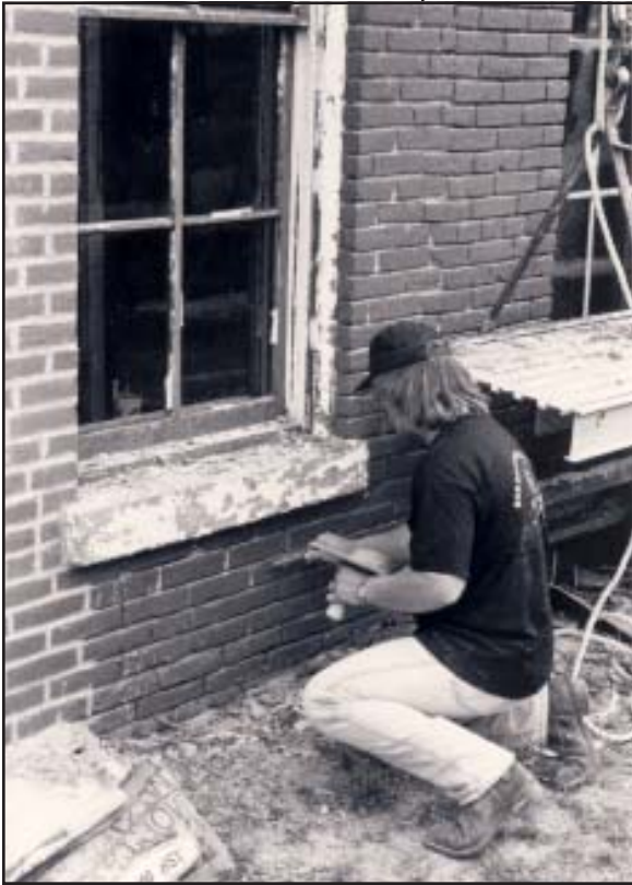
Brick Mason Bob Bohot inserts new soft mortar into recently raked mortar joints at the Joseph Inslee house, 524 N. 6 th Street, Robidoux Hill Historic District
