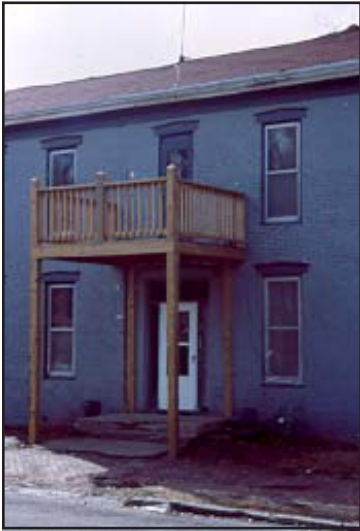
Paint all visible porch features. Treated materials, when used, should be painted following a proper period of drying/curing.
