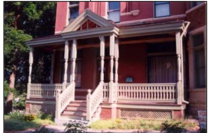
The newly reconstructed front porch on the August Nunning house, 1401 Jules Street, Museum Hill Historic District, rests on brick piers that are in-filled with frame lattice panels in the traditional style.
